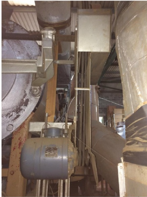
Figure 6: The motor pulley system used to rotate the roasting drum
