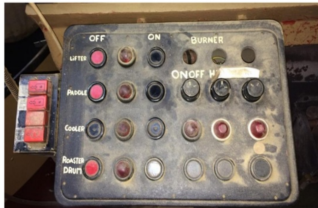
Figure 4: The existing control console.
