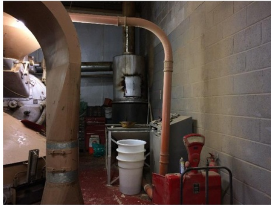
Figure 3: The riser pipe off the blower
