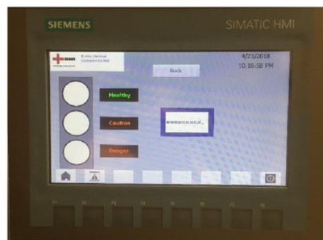
Figure 55: Shows the alarm screen of the roasting drum temperature alarm condition
