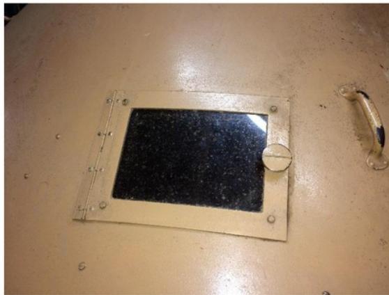
Figure 8: Shows the access hatch used to check the bean temperature.
