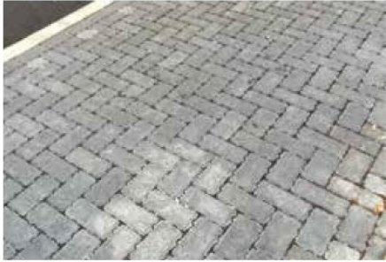
a Block permeable paving
