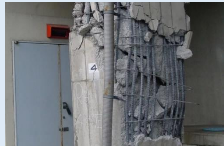
Figure 6. Column failure due to inadequate amounts of fine aggregate (Articles, 2020)
