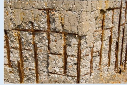
Figure 5. Reinforced steel corrosion (RUSTX CCI, n.d.)
