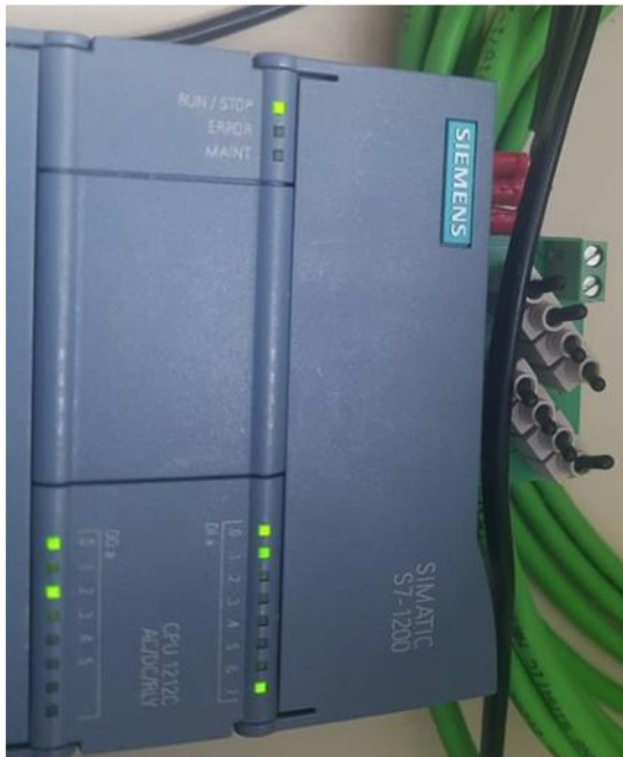
Figure 36: The outputs set on the PLC and the inputs being received from the webpage.
