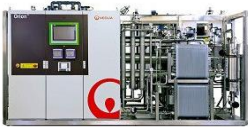
Orion Purified Water Generation Plant. Photo courtesy of Veolia Water Technologies
