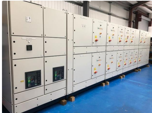
Figure 1 - Form 4 Motor Control Centre
