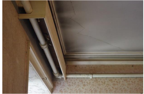
Fig 59 Room 4: House Keeper's Room, Cornice and pipes.
