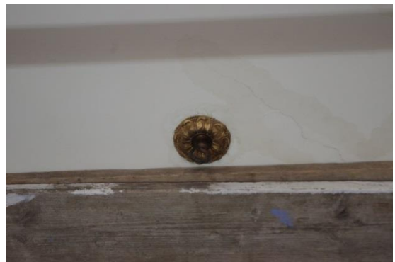
Fig 109 Room 8: Saloon, light fitting.
