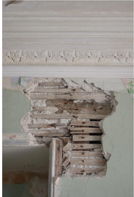
Fig 141 Room 11: Pink Bedroom, missing plaster and cornice in south wall.
