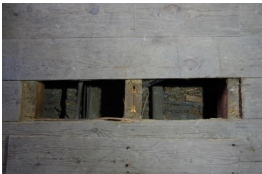
Fig 183 Room 15: Lifted floorboard in Attic Gable Room.
