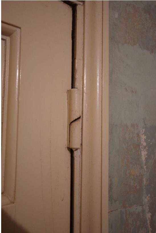
Fig 157 Room 13: Dark Room, door hinge.
