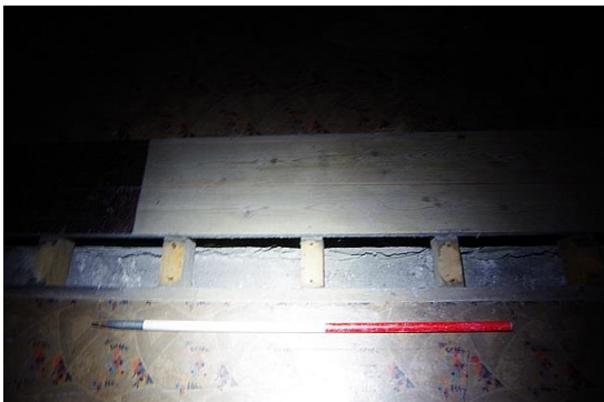
Fig 176 Room 4: Raised floorboard in House Keeper's Room.
