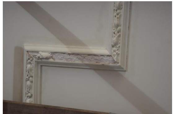
Fig 108 Room 8: Saloon, ceiling showing damaged ribs.
