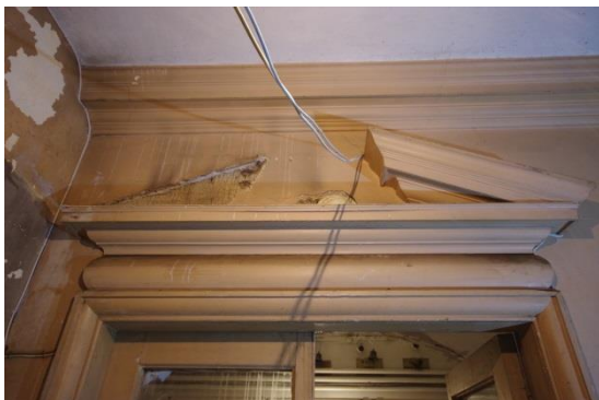
Fig 39 Room 1: Detail of broken pediment over door opening in south wall.
