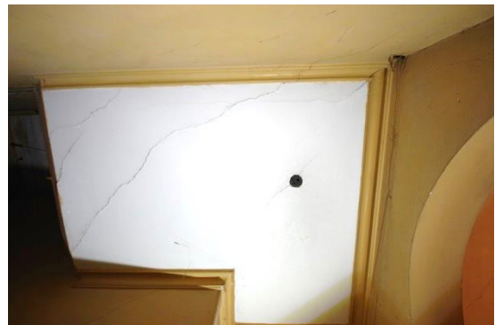
Fig 41 Room 1: Ceiling at the base of the stairs.
