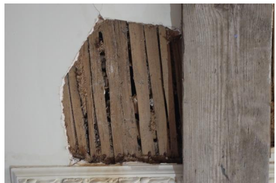
Fig 110 Room 8: Saloon, missing plaster in ceiling.
