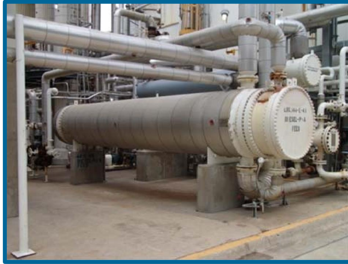
Figure 20: Typical Refinery Shell and Tube Heat Exchanger (Valero Energy Ltd, 2017)
