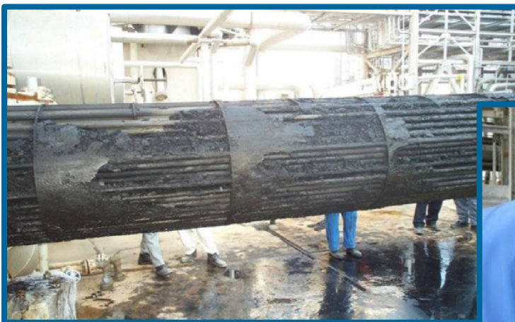
Figure 28: Shell side baffle fouling (INTECH, 2018)
