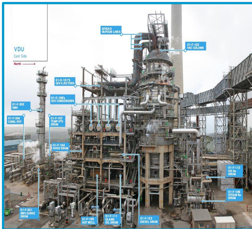
Figure 5: Vacuum Distillation Unit including main vacuum column (Valero Energy Ltd 2018).
