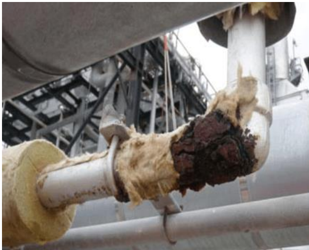
Figure 4.1 Localised CUI on pipework (BoilerRock, 2017)
