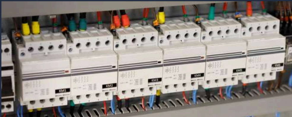
Industrial bank of relays
