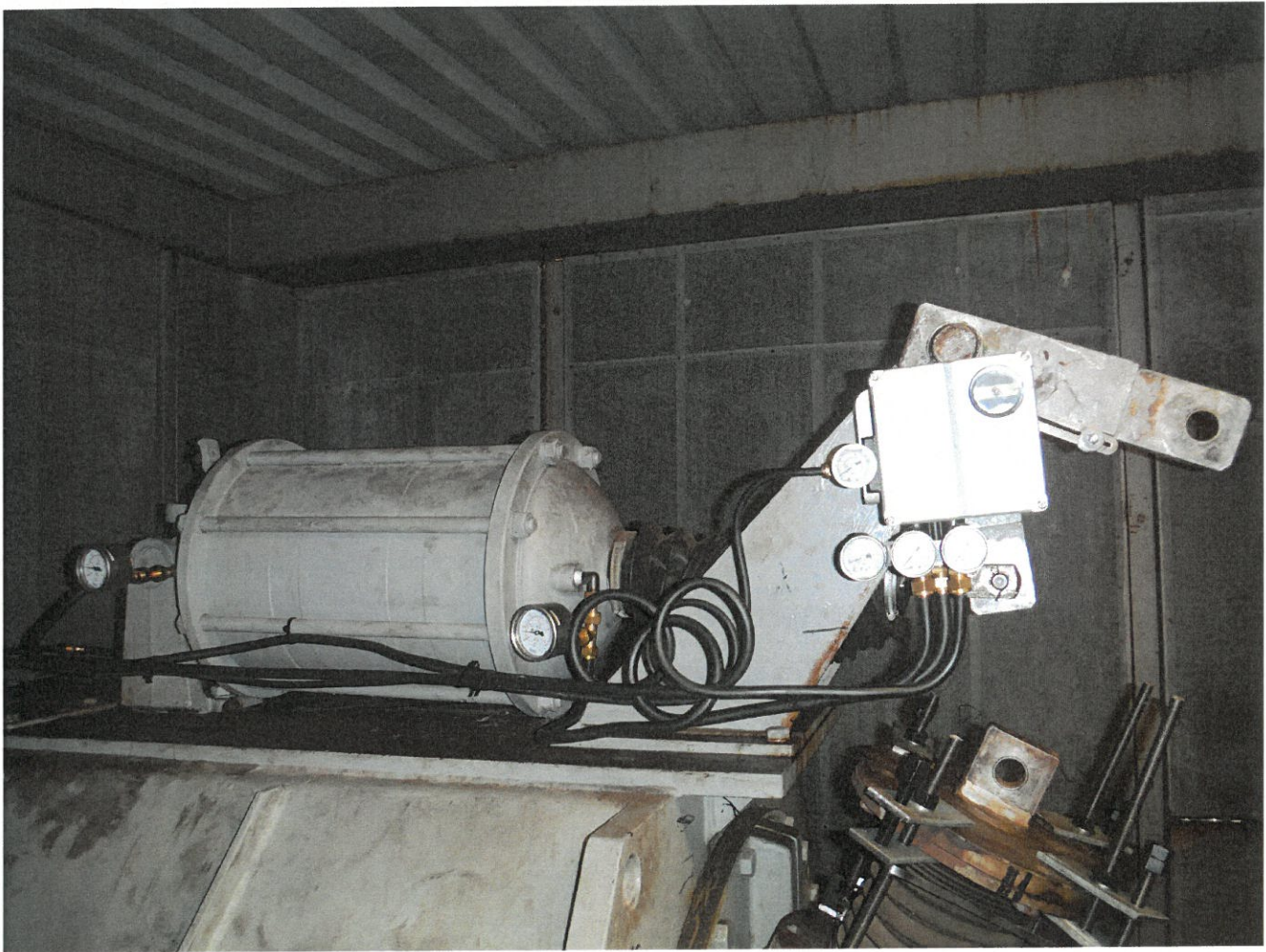
Figure 3, Source: Heather Raymond, Valero Refinery Date?
