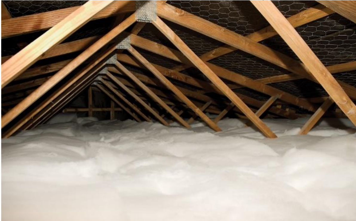
Figure 7: Blown Fibre Insulation. Source: (Mammoth, 2017)
