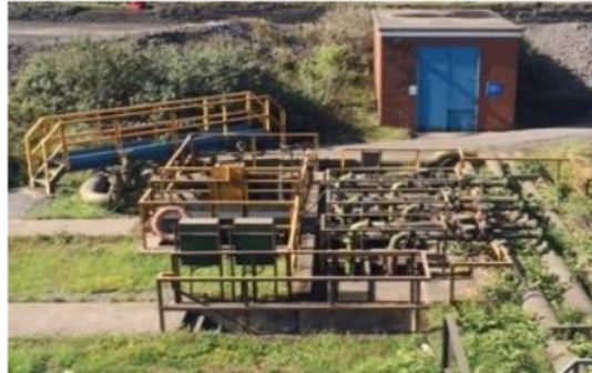
- The Arnallt Contactor room and Sump area containing the 8 pumps
