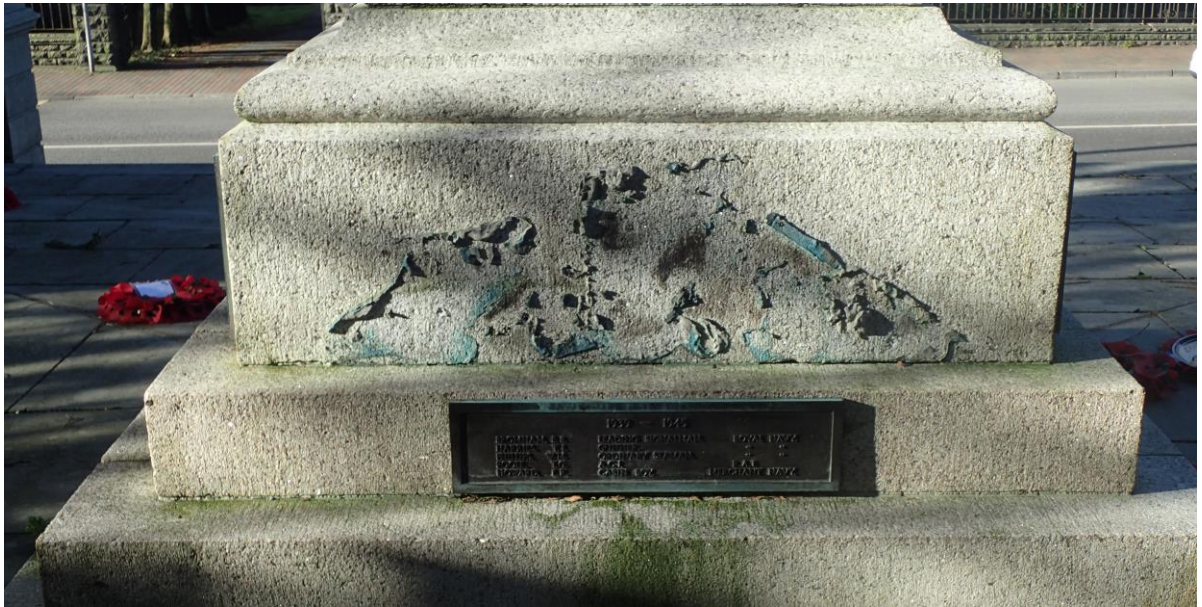
[Damage to the rear of the Briton Ferry War Memorial, Z. Bridges, 2018.]
