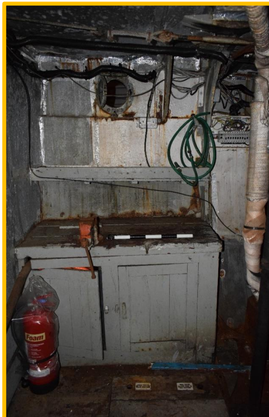
Figure 22 Work bench in engine room
