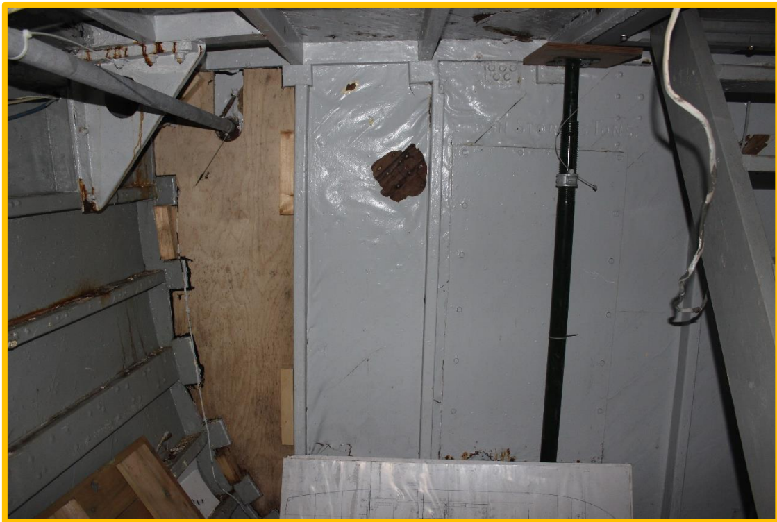
Figure 26: Bulkhead at frame 22, with brown rot
