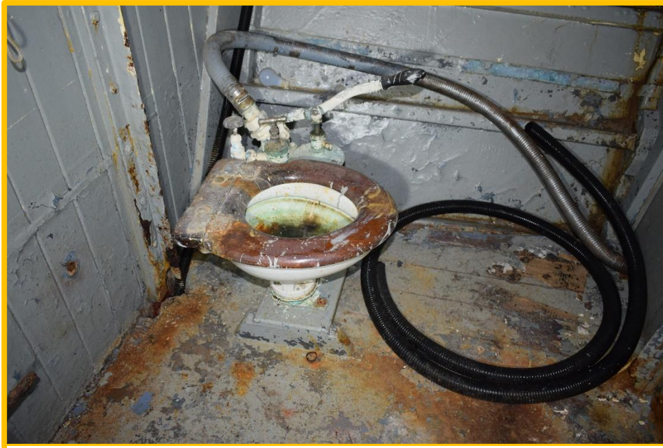
Figure 16: Blake toilet on RML 497
