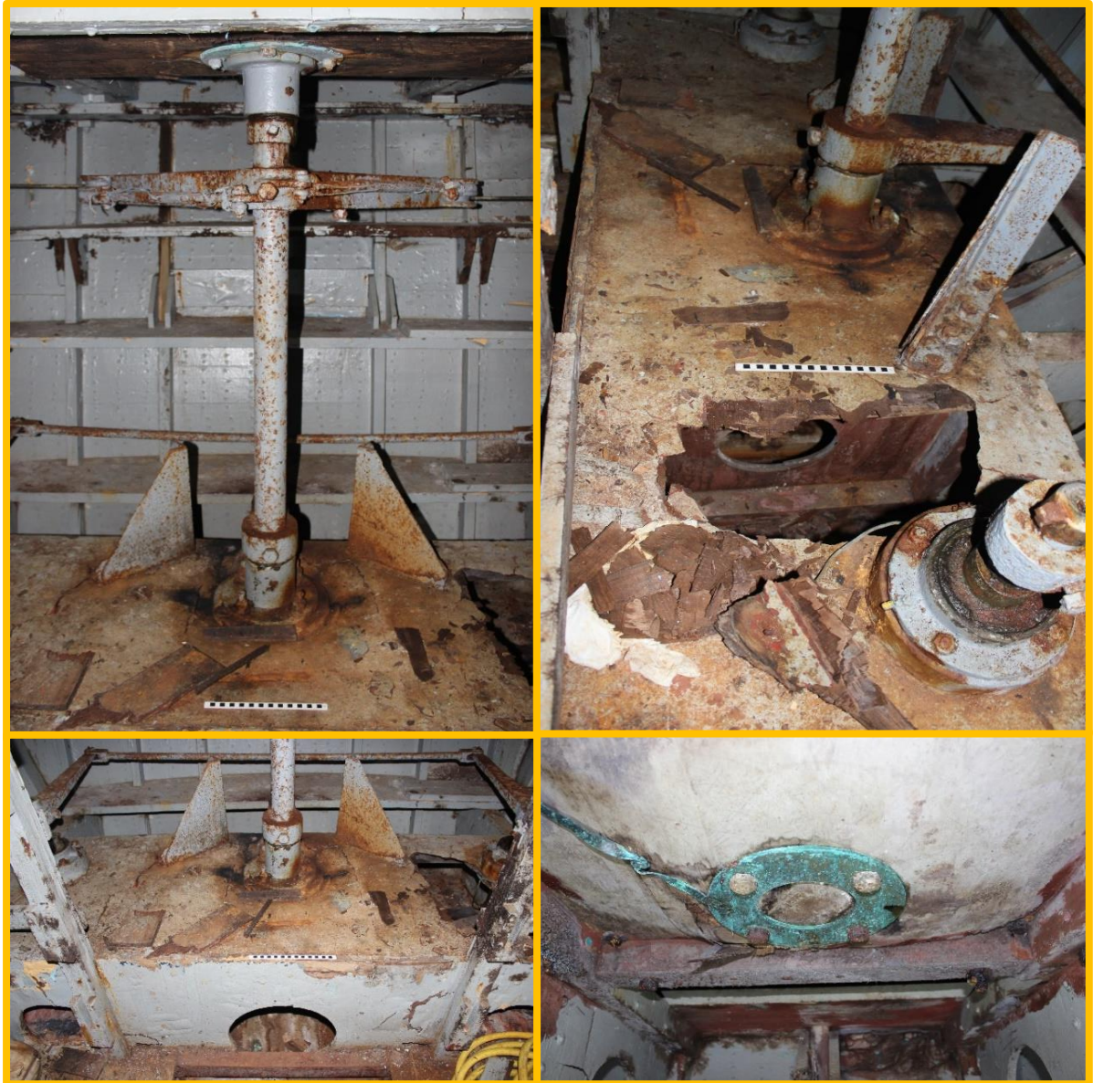
Figure 28 Top to bottom, left to right: Steering quadrant on plywood box; hole on the port side of the plywood box; plywood box sagging beneath weight of the steering gear; underside of plywood box showing lack of support
