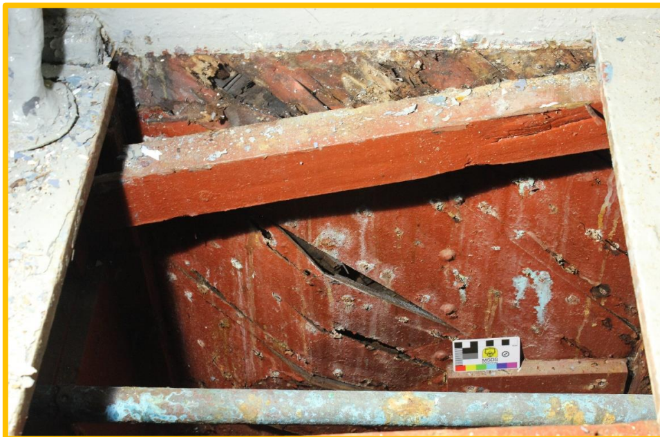
Figure 10: Buckled section of bulkhead 4, forward face, port side.
