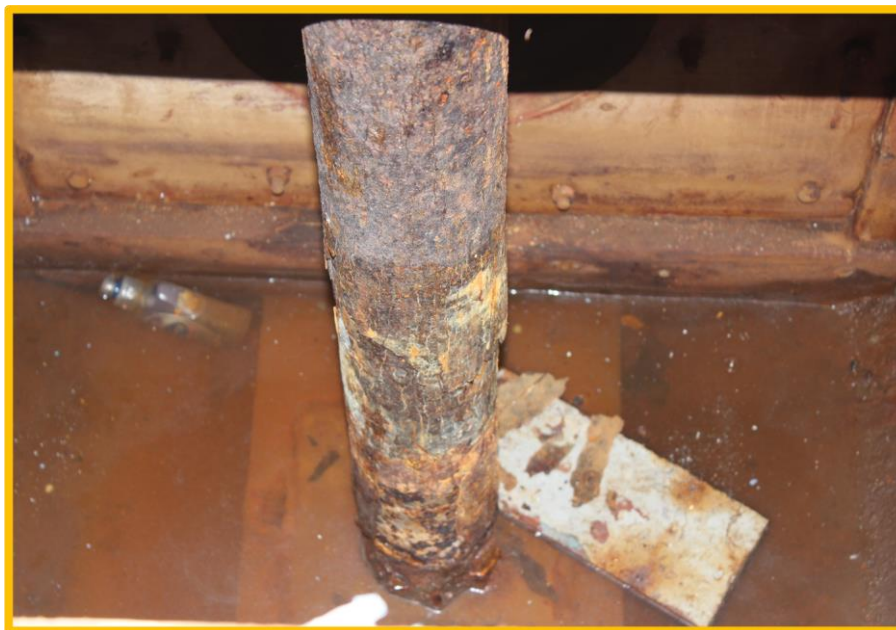
Figure 11: Base of large metal support with close up of support in bilge water below decks
