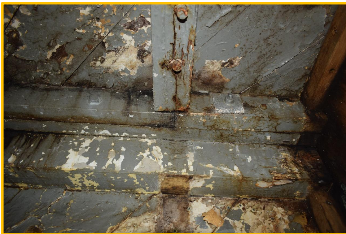
Figure 7 Beam shelf between frames 9-10 on starboard side, with dry rot
