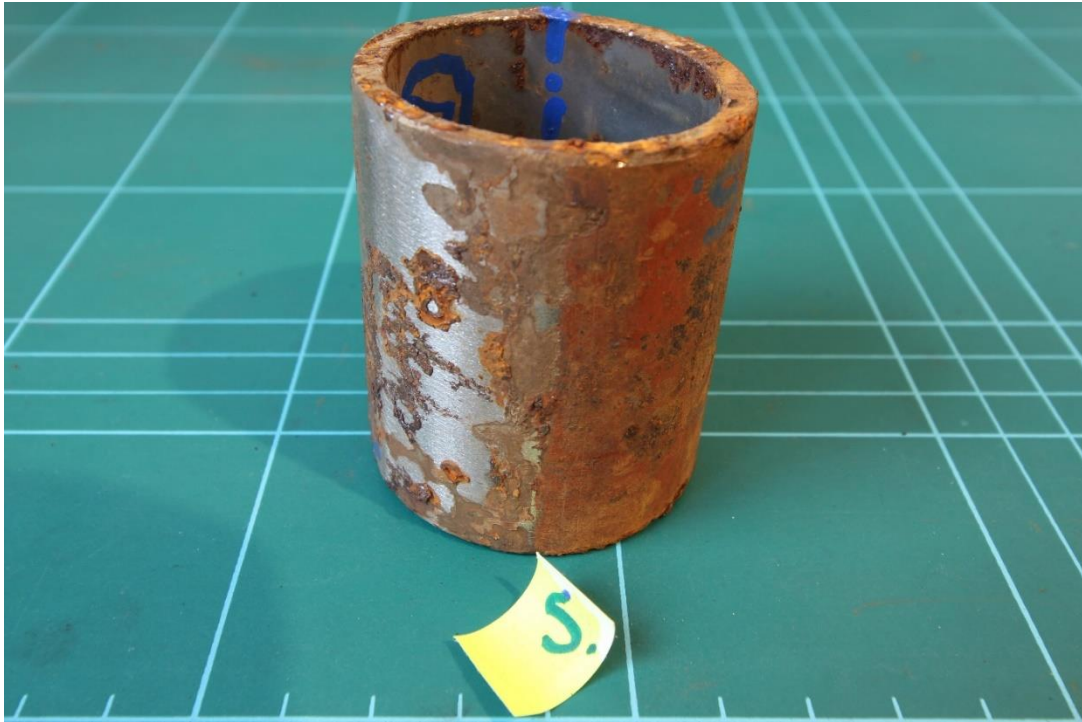
Figure 4.28 Pipe Sample 5 Ambient – Glass wool insulation - Lower 180°
