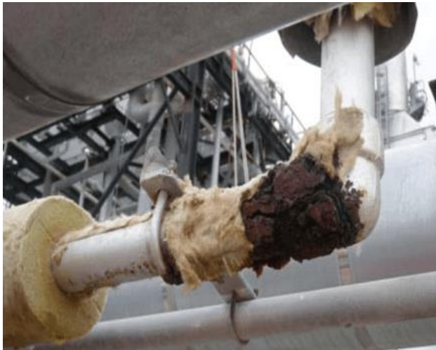
Figure 1.1 Localised CUI on pipework (BoilerRock, 2017)
