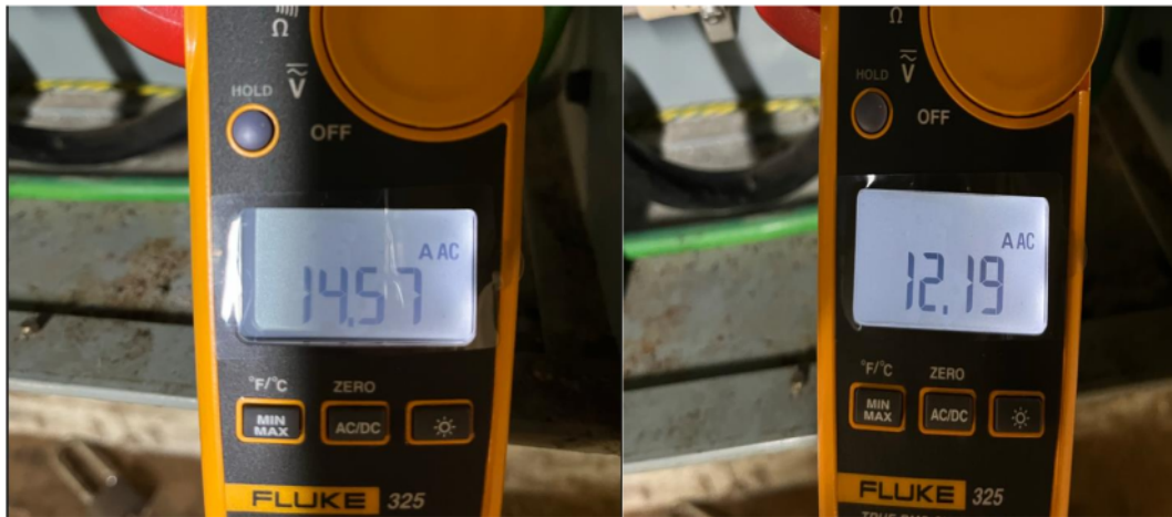
Figure 6 - Motor 1 & 2 Current Readings
