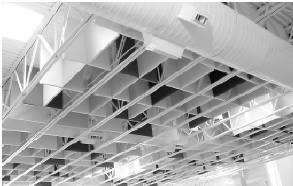
Indoor HVAC System, (Photo courtesy of Water Technology, Inc.)
