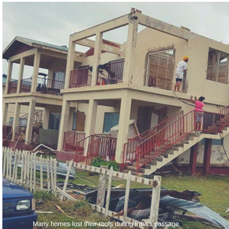
A family home lays in ruin after Irma
