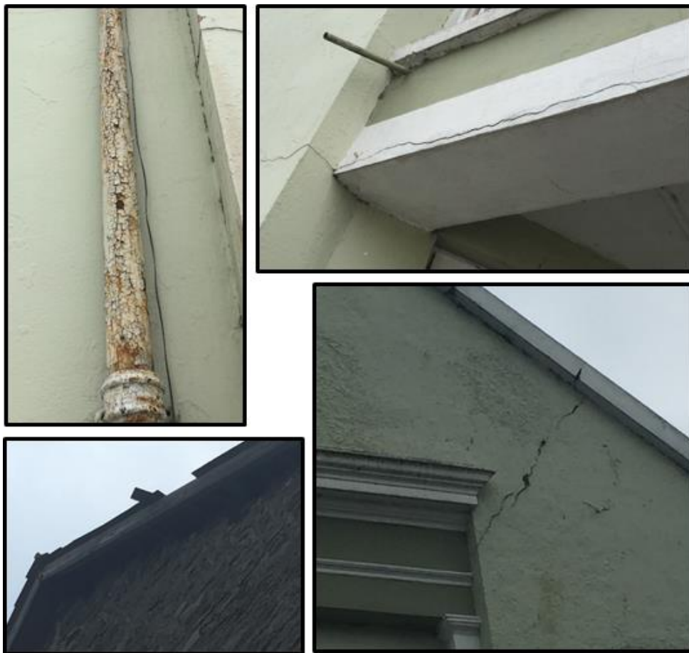
Figure 8 = Required Maintenance & Repair to Victoria Hall. Giles, 2019
