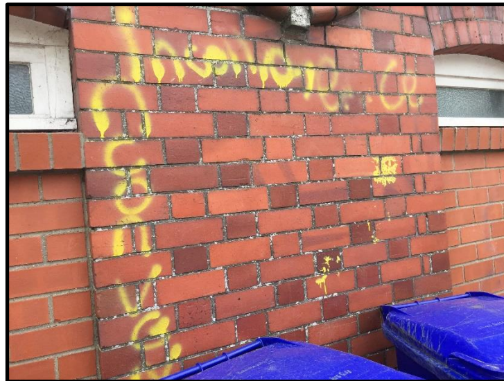
Figure 14 = Vandalism on the toilet exterior. Giles, 2019
