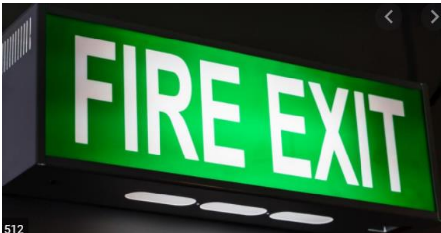
Figure 16: Common emergency lighting signage: Safelincs, 2020
