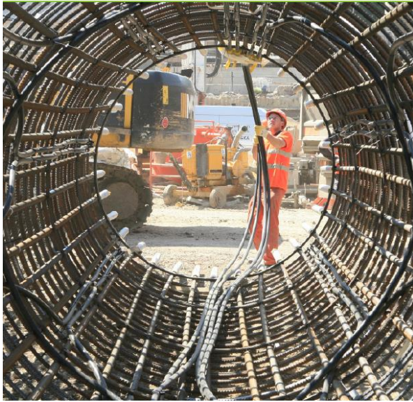
Figure 13: Green solution energy piles SKANSKA
