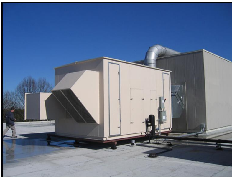
Figure 4: Roof mounted Air Handling Unit (AHU) Indoor Air Quality, (Natel, 2020)
