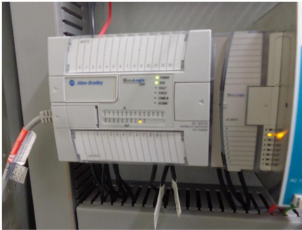
FIGURE 43 - PLC DURING TESTING
