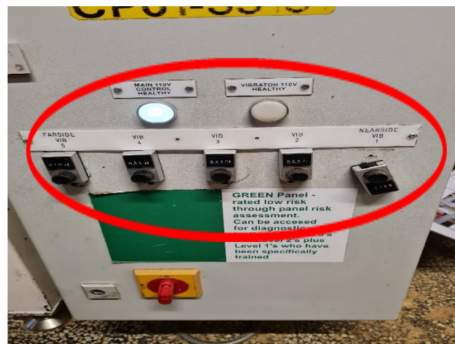
Figure 26- Damaged speed controllers.
