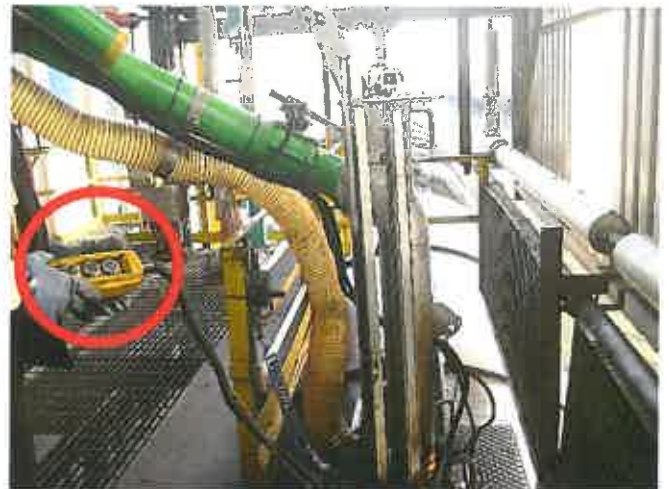
Figure 5. This shows a loading arm in place. All arms are controlled by a pneumatic system and the control pad circled in red is used to manoeuvre the arms up and down.
