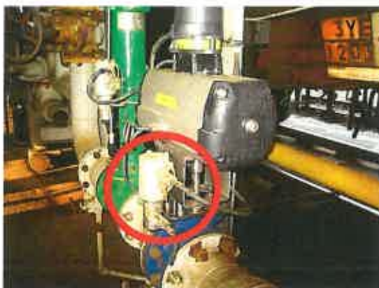
Figure 3. This shows one of the SIS valves that must be in the open position before any loading can commence on the Rail. This also illustrates the SOV which can be used to manually open or close the valve, this SOV is connected to a safety PLC. These valves are controlled by a pneumatic system, supplied from compressors, if the air fails, it will fail shut to prevent any loss of containment.
