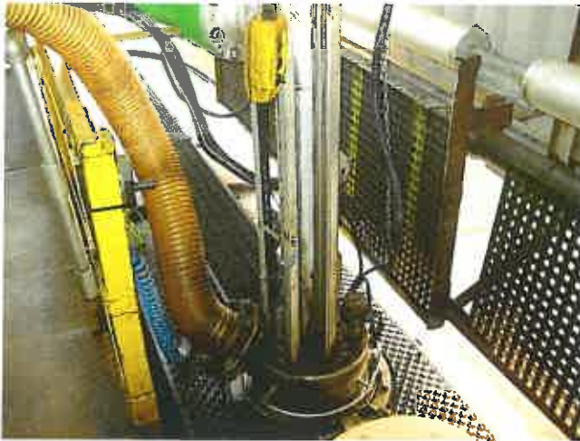
Figure 12. This illustrates a loading arm ready to go, with the correct earthing, high level probe down and solenoid valve open. Once these 3 steps are done, the meter head will display a start permissive, enabling Operators to commence loading.
