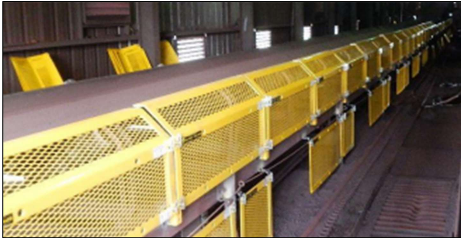
Figure 5 - Machine Guarding Example on a Conveyor, Courtesy of (Dirgie & Duffy, 2019)
