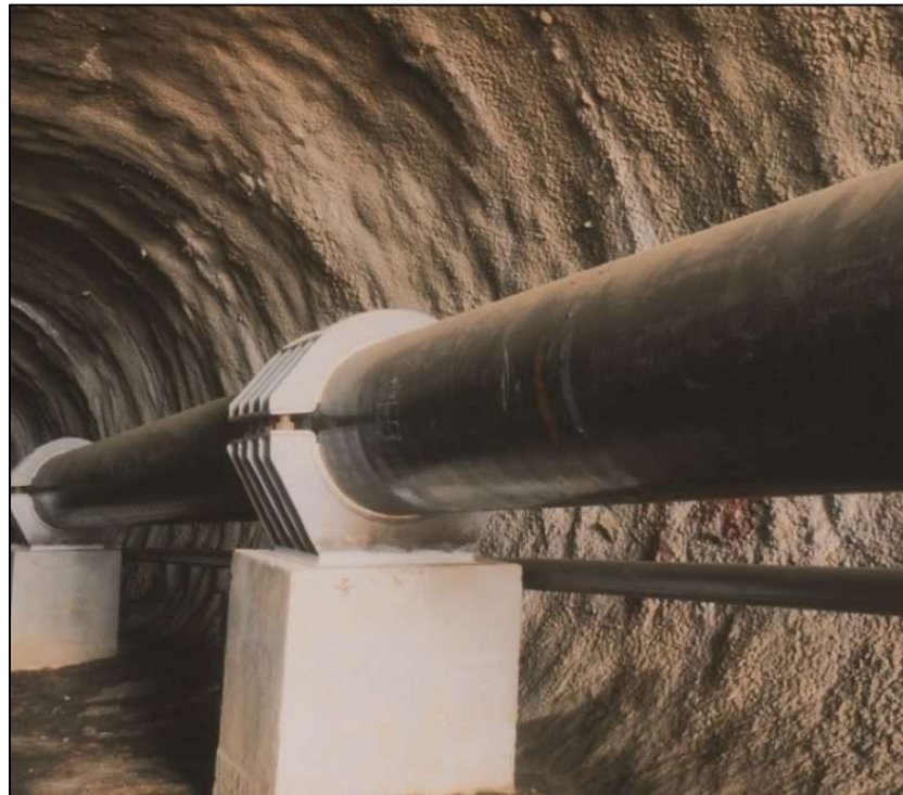
Figure 7 - Example of Underground Slurry Pipeline in Minas-Rio, Brazil, Courtesy of (McKay, 2018)
