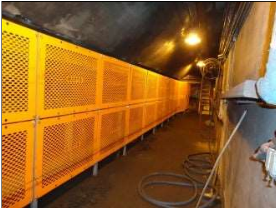
Figure 6 - Alternate Machine Guarding Example on a Conveyor, Courtesy of (Rowland, 2014)
