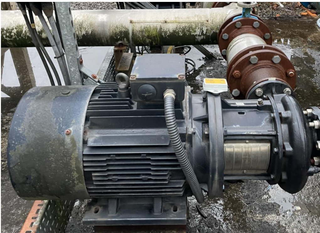
Figure 31. Chiller pump with BoB sensor installed (Tauseef, 2024)
