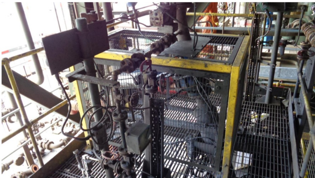
Figure 2.4 – Machine guarding in place around PV345
