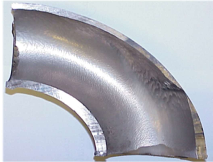
Section view of a metallic pipe that has experienced erosion. ResearchGate.net, 2018 )
