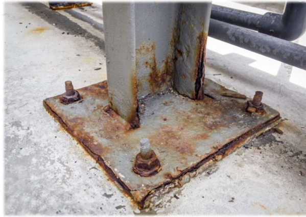
Photo of a piping support base plate (Corbett.N, 2021)
