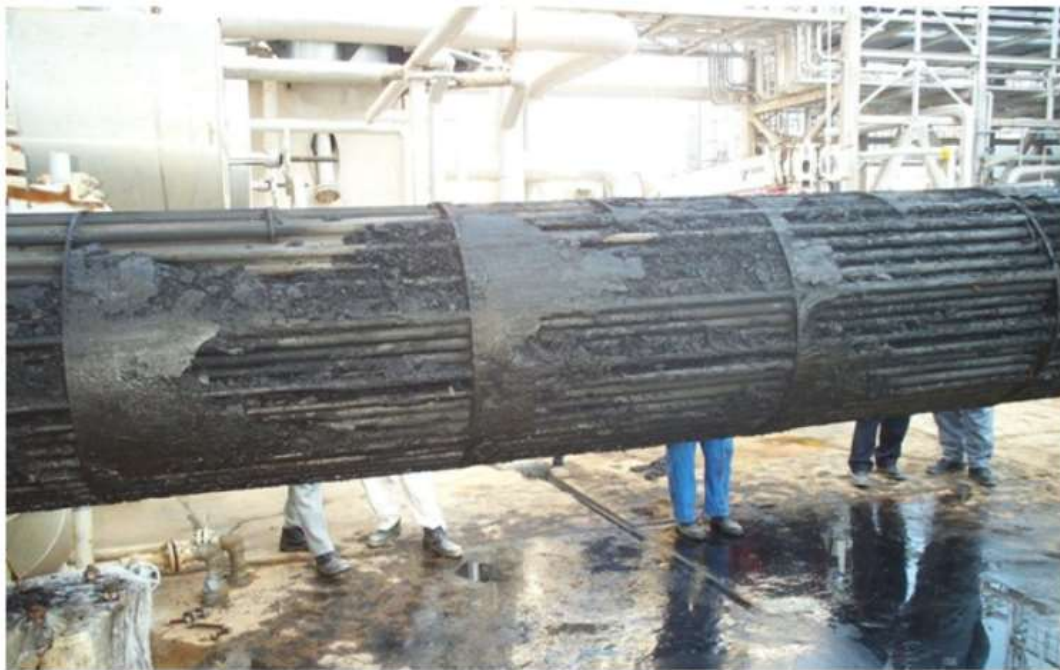
Image depicting fouling of a heat exchanger. ( Intechopen.com,2023 )
