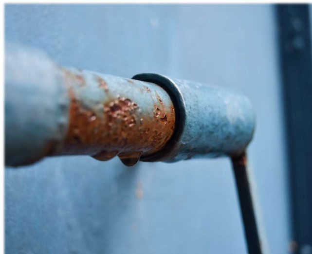
Photo of a pipe that has experienced corrosion. (Corbett.N, 2021)
