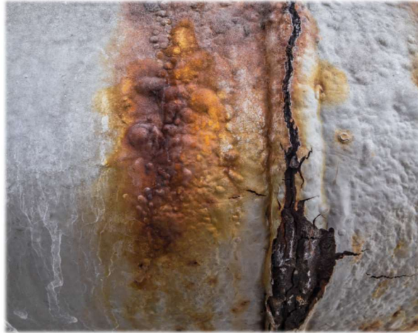
Photo of the outside of a pipe that has suffered stress cracking corrosion. (Azom.com, 2001)
