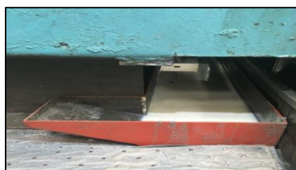
Figure 21: Strategical Placement of Individual Drip Trays
