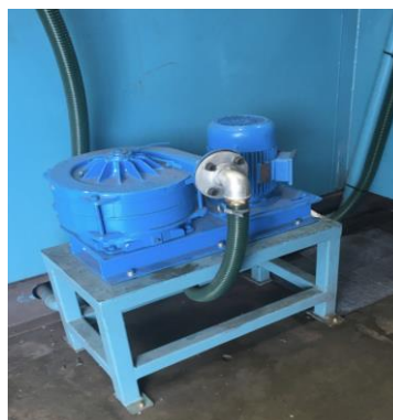
Figure 28: Compatible Centrifugal Pump Installation and Trial
