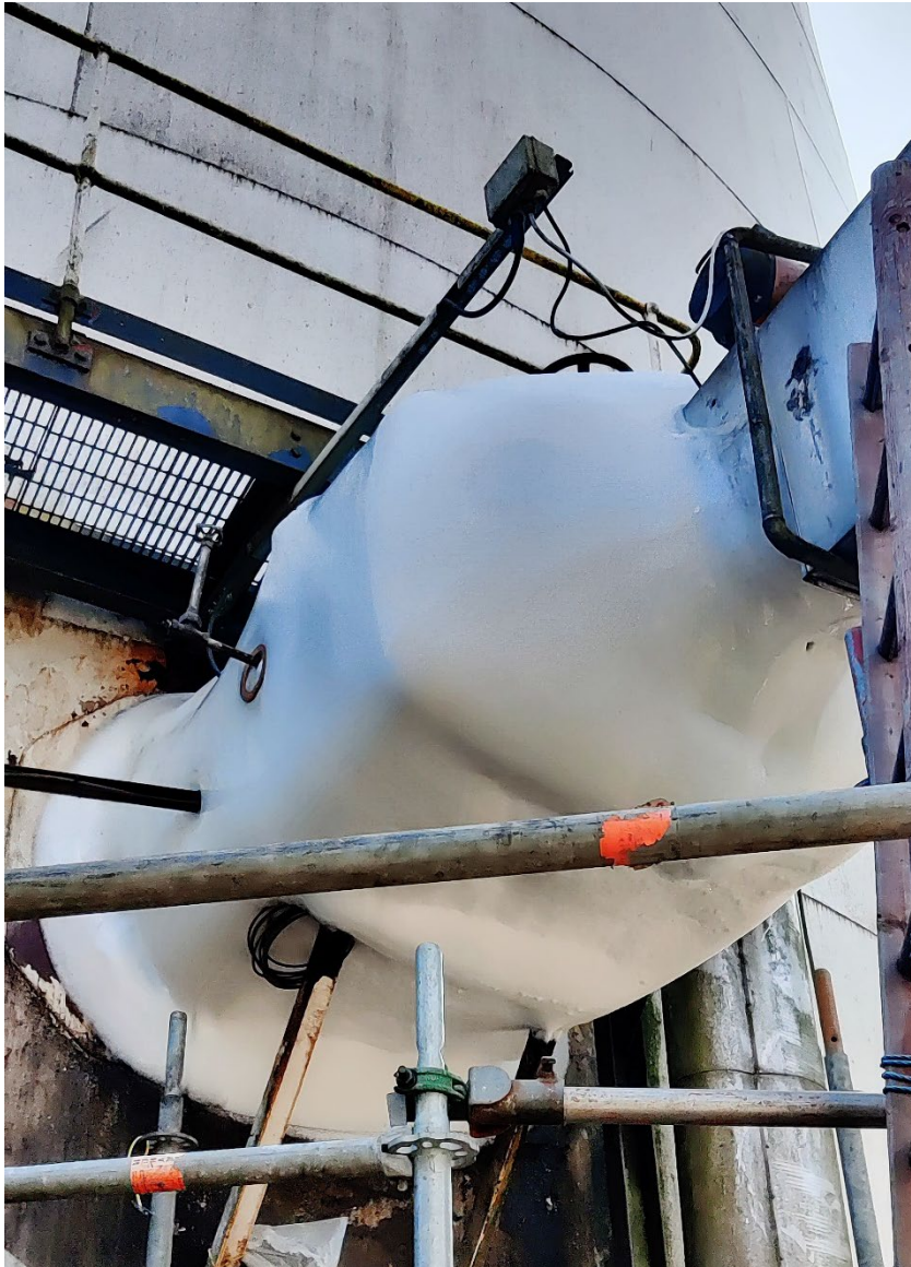
Figure 7 BOC actuated nitrogen valve (Iced up)
