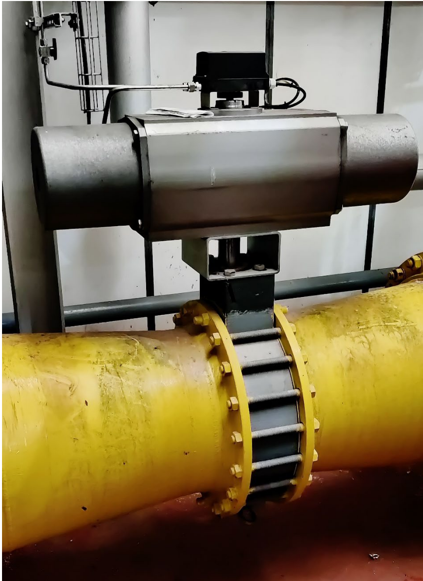
Figure 3 BOC actuated valve in Air service
