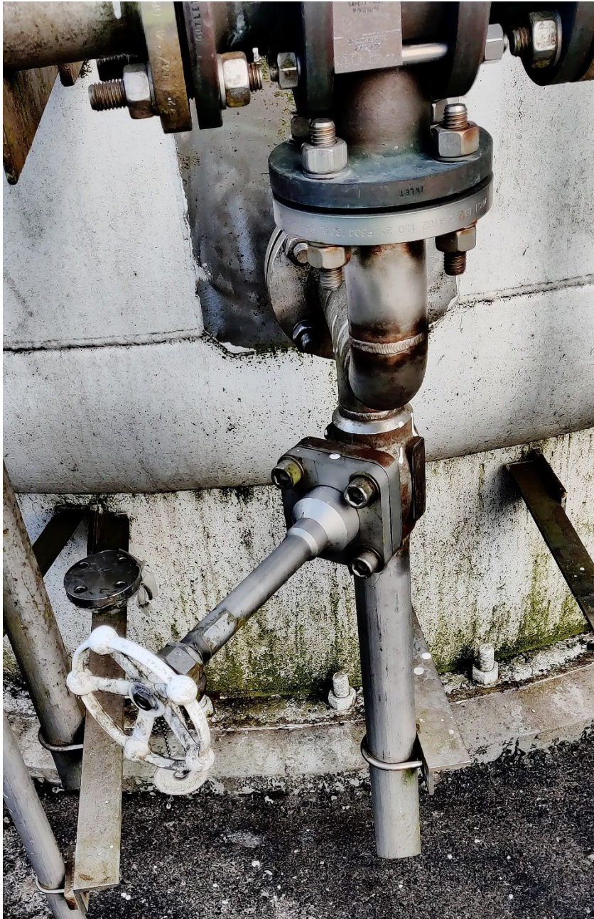
Figure 6 BOC Oxygen manual vent valve
