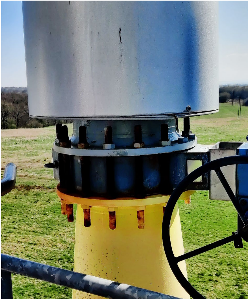
Figure 4 BOC Butterfly valve in Air service
