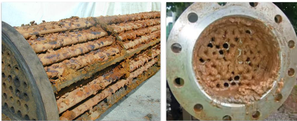
Figure 4:Fouling in shell and tube heat exchangers.
