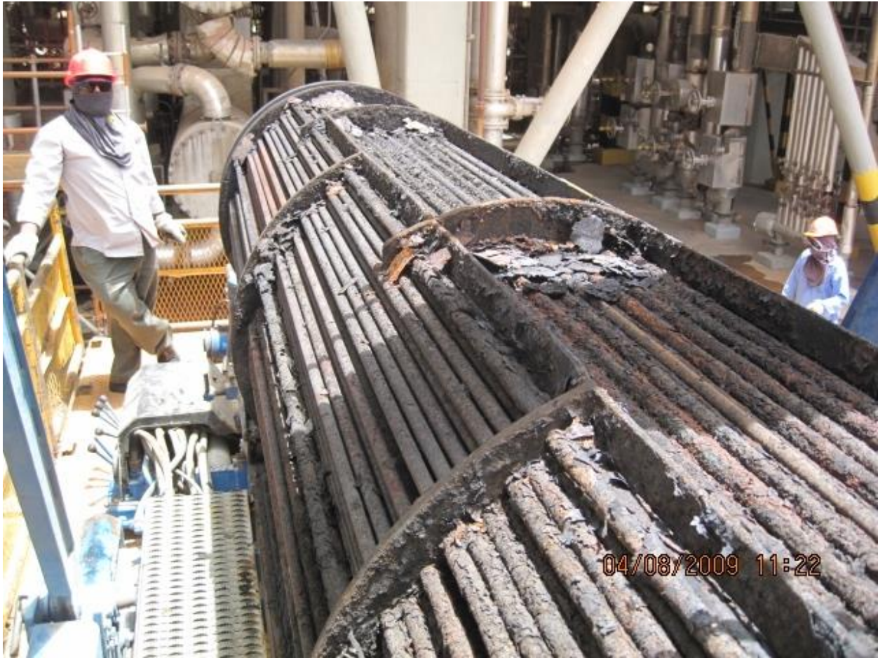
IMAGE - 2 Fouling in Shell in Tube Heat Exchanger
