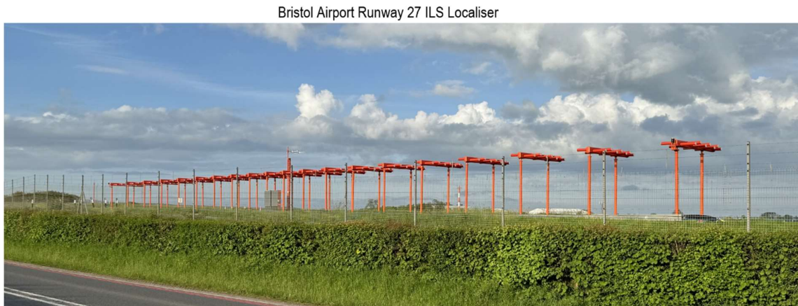
Figure 53 Bristol Airports 27 ILS Localiser (Lewis, 2024)
