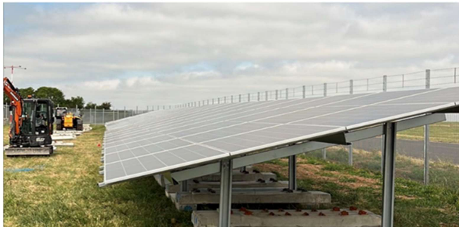
Figure 6 Bristol Airport's New 1.4MW Solar array (BRS, 2024)
