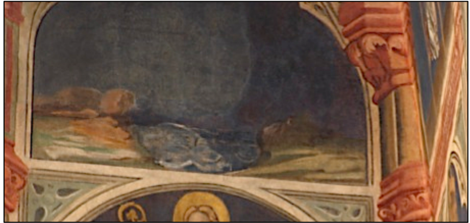
Figure 52. The damaged image at 99A at the end of the south wall, top register, south wall, Salone, Palazzo della Ragione, Padua. Photo: D. Gunzburg.
