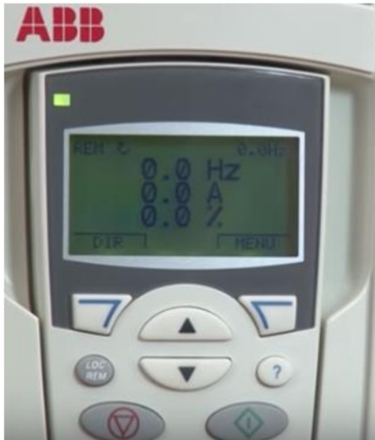
Figure 17: ABB drive set up
