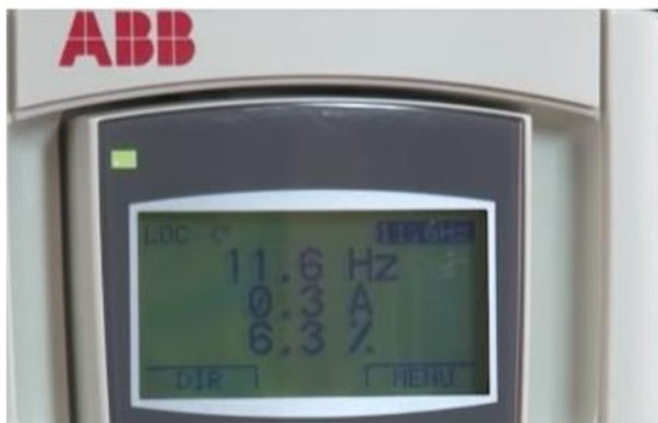
Figure 36: ABB drive test
