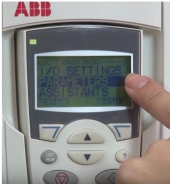
Figure 18: ABB drive set up
