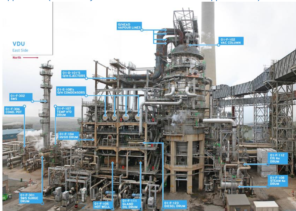
Figure 25 01-VDU Shown from east side of unit
