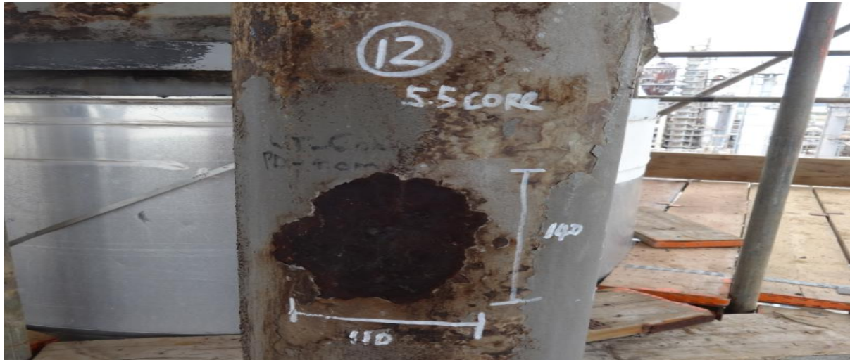
Figure 6 Corroded section of 01-WP-3017-8" at location 12 with 0.5mm remaining wall thickness
