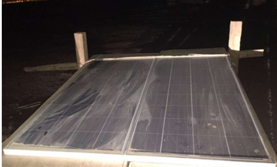
Figure 16: live photo for the tested PV-solar panel.
