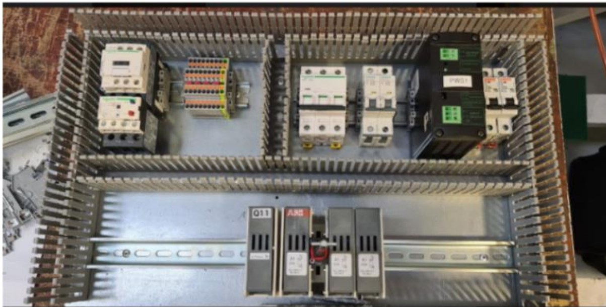
Figure 25 Electrical Panel Before wiring
