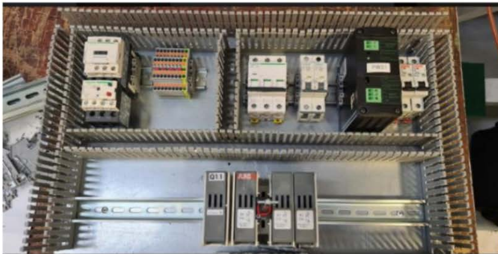
Figure 25 Electrical Panel Before wiring
