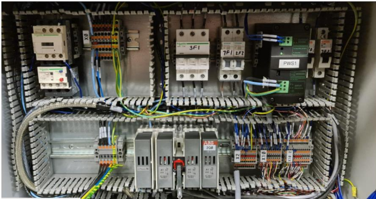
Figure 26 Electrical panel complete
