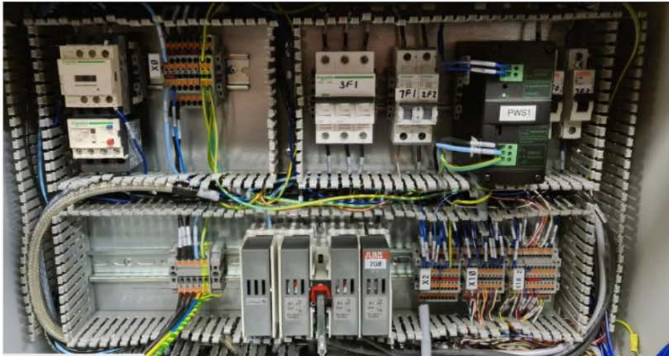
Figure 26 Electrical panel complete
