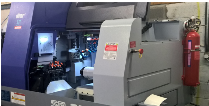
Fig.4 Star Lathe with Fire Trace system integrated
