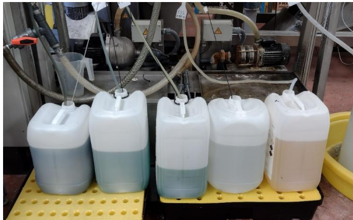
Figure 6 - 5 Chemical Tanks Beneath the Pumps
