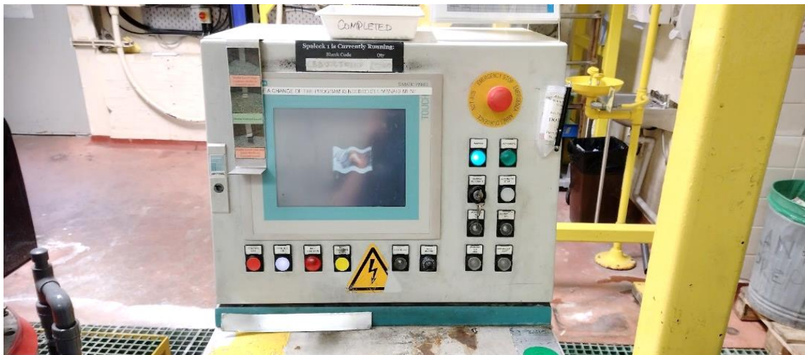
Figure 10 - HMI, Positioned at the Right Side of the Machine
