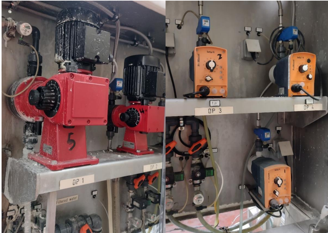
Figure 8 - 5 x Existing Pumps
