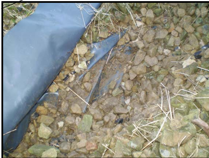
Photograph 5 – Showing Membrane and Excavated Aggregate Demonstrating No Visible Sand Blinding Next to Membrane
