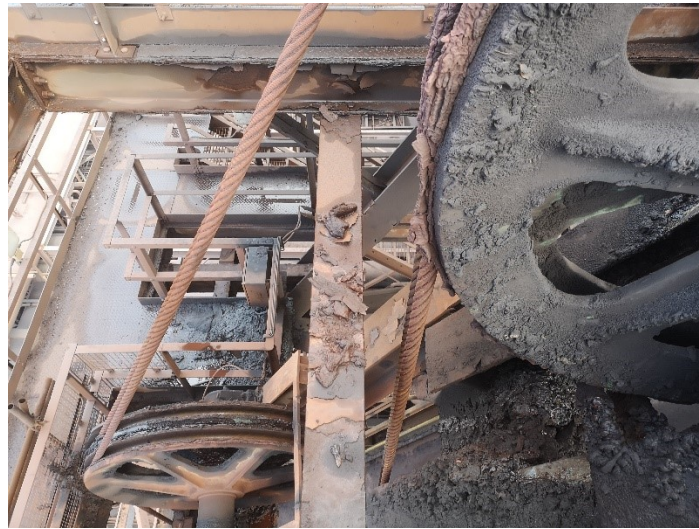
Figure 37 - Evidence of poor cleaning/lubrication
