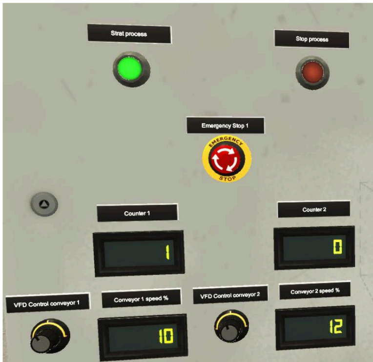
Figure 48 - Panel Speed Set at 10 and 12 for Conveyors 1 and 2
