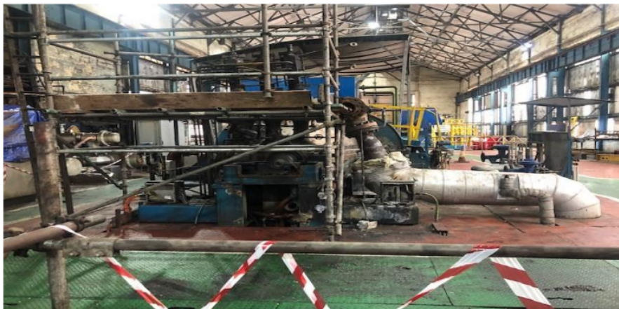
TA9-Turbine Hall shortly after the incident in 2021 (fig 3)
