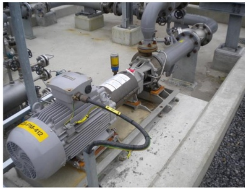
Figure 17 - Motor being ran with coupling dropped
