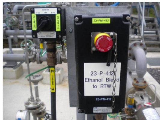
Figure 15 - Control at motor
