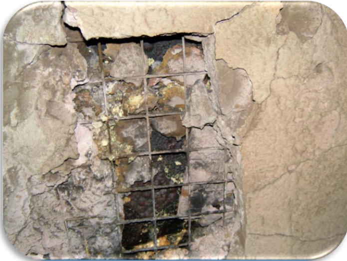
Figure 22: Vibration induced refractory damage resulting in localised casing hotspots
