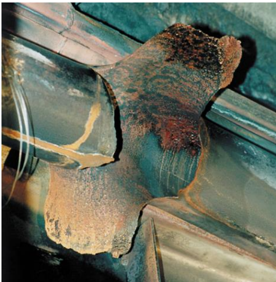
Figure 4: Tube rupture (Babcock & Wilcox, 2017)
