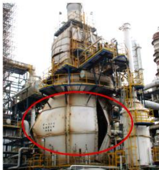
Figure 5: Furnace distortion (Wu, 2019)
