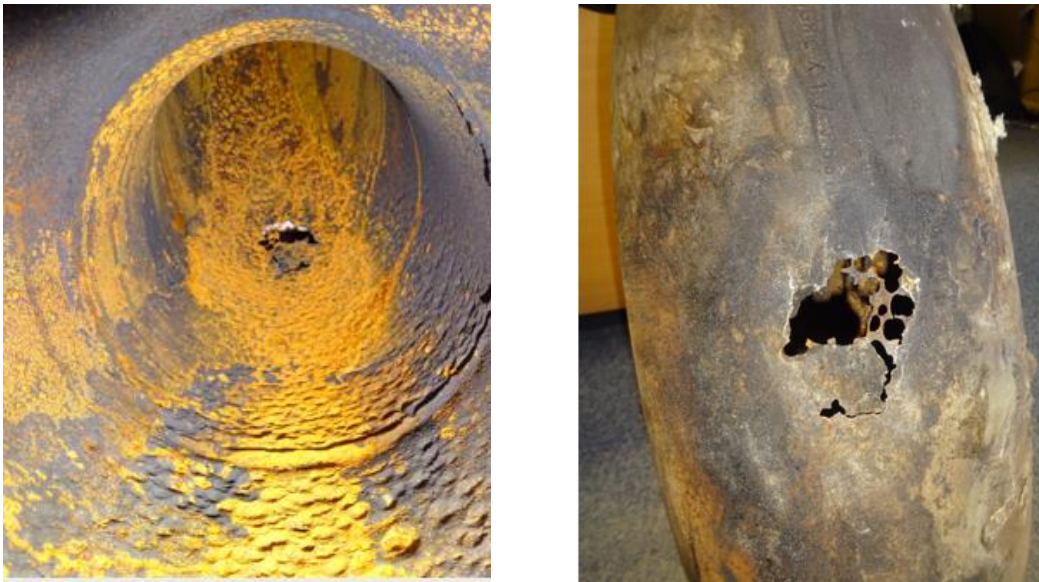
Figure 8/9: Tube failure due to accelerated erosion
