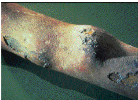
Figure 10: Tube bulge (Babcock & Wilcox, 2017)
