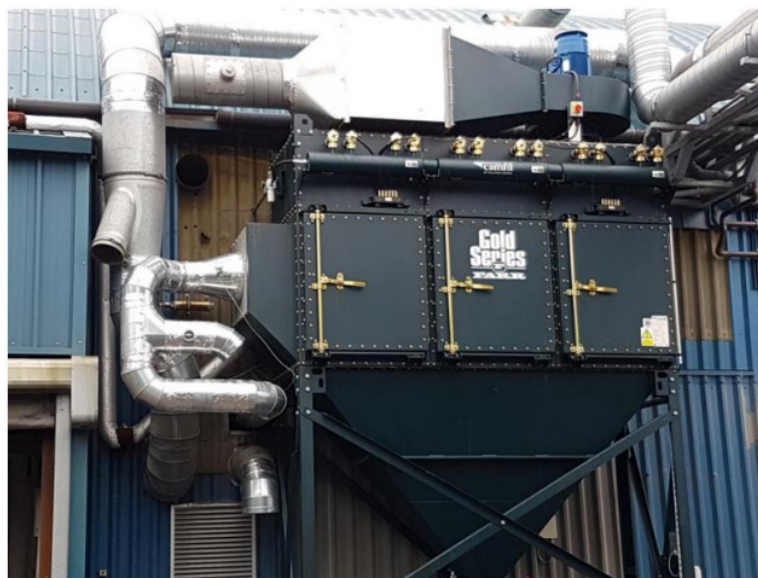
Figure 1 - Atomising Plant Dust Collector
