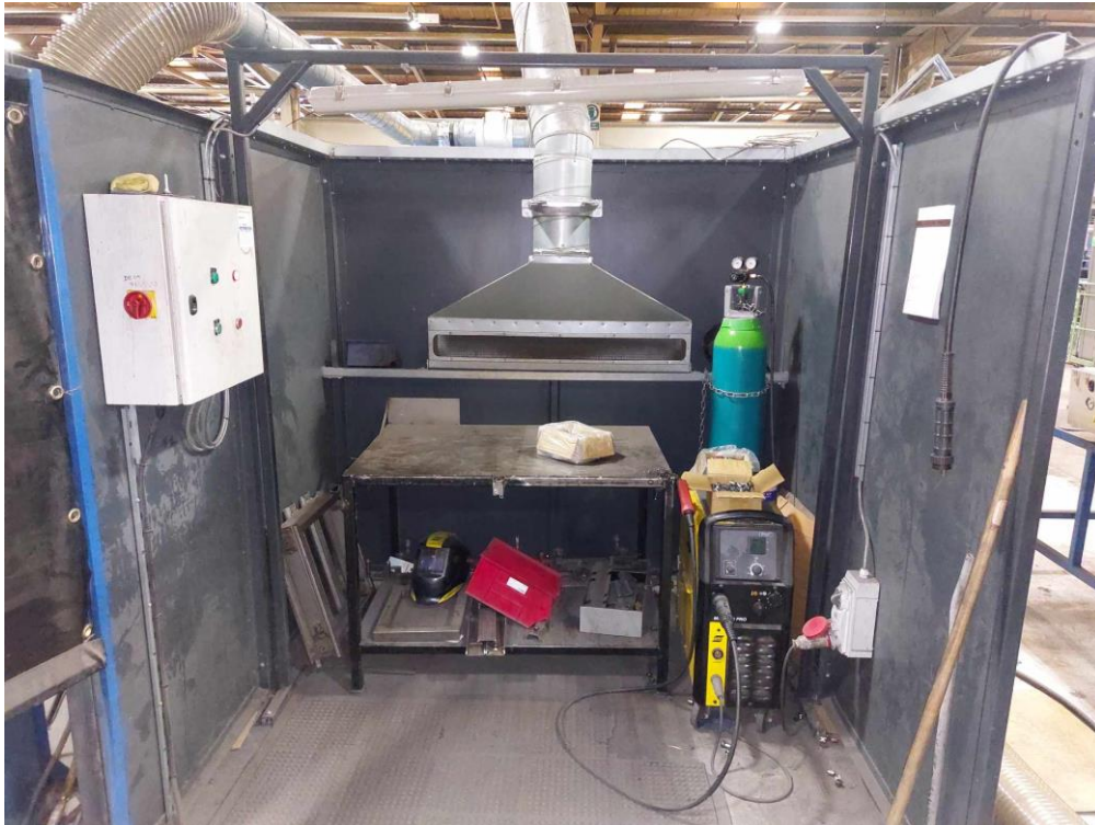
Figure 12- Welding Bay with New Control Panel
