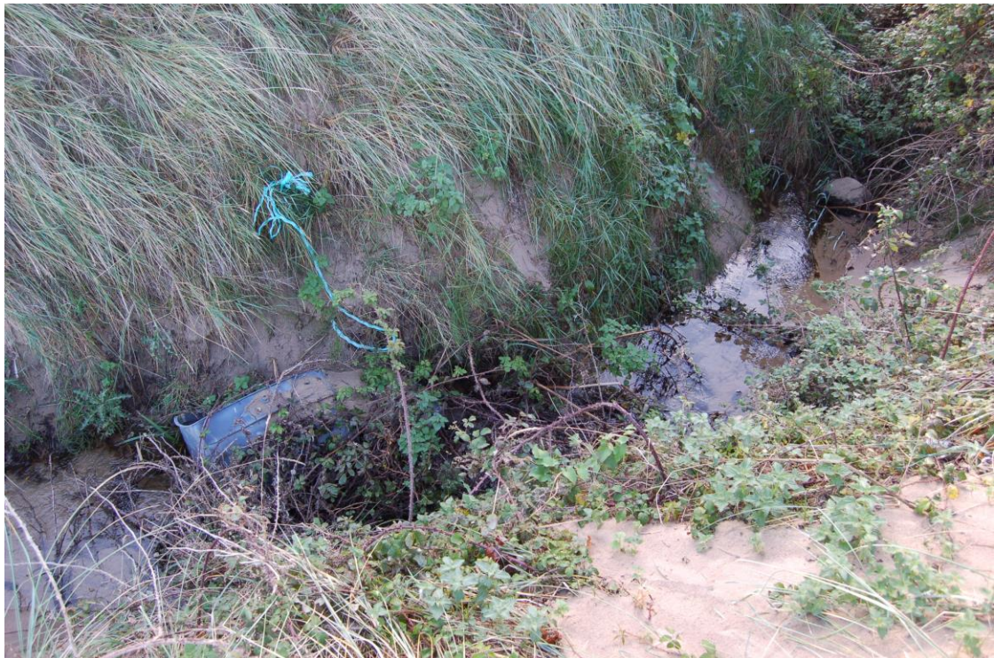
Some debris that collected at the outlet to the beach
