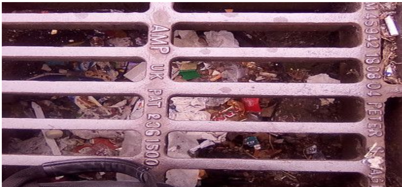
Business district Birchfield Road in Perry Barr Birmingham. Cause of blockage to the water system by plastic pollution.
